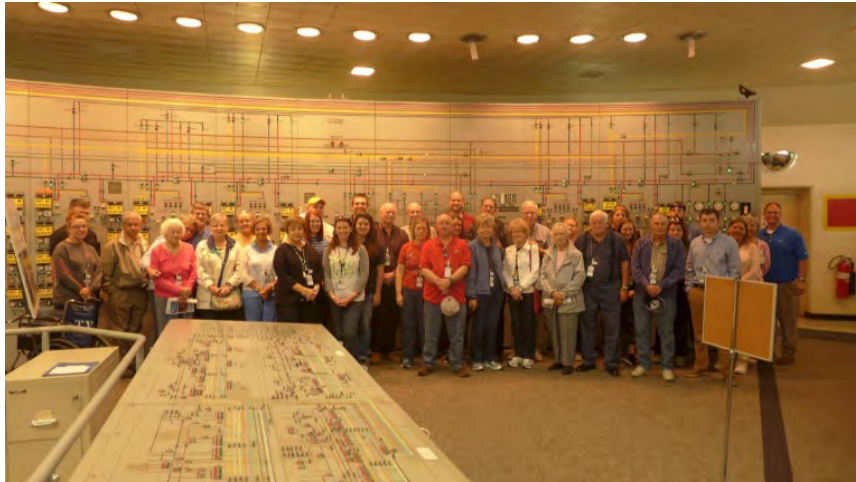
Figure 3.2 Participants in the inaugural PGDP Site Tour visit the C-300 Central Control Facility
